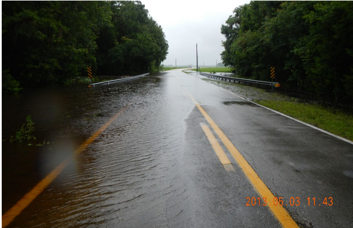
Figure 94 CR 13N Flooding During May 3, 2013 Rainfall Event
