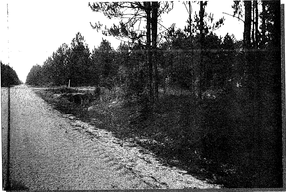
Heavy rains swell the drainage ditches to overflowing levels causing erosion and additional costs for maintaining traversable roads.
